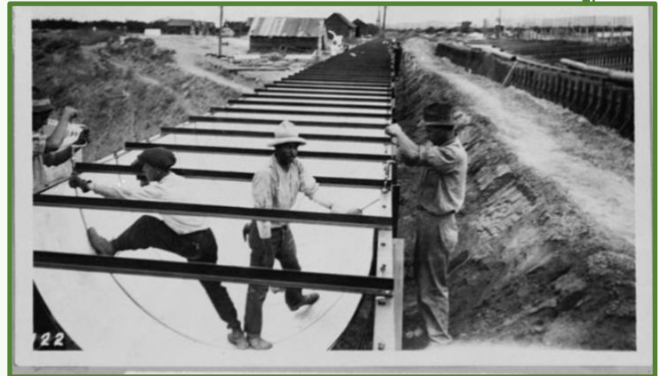
Tightening joints and adjusting plates on steel flume at Mockingbird Dam on the Gage irrigation canal. Photo credit: Library of Congress
